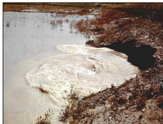
Figure 4-15. Photograph of a whirlpool along the upstream slope of an embankment dam.
