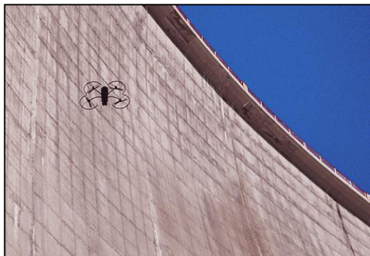
Figure 8-4. An inspection drone at work photographing the downstream face of the Tseuzier Dam in Valasi, Switzerland.
